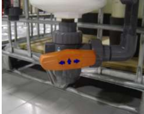
Figure 4: V9 in Position 1
