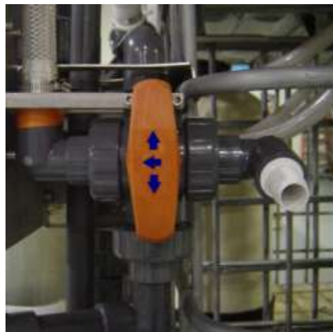
Figure 3: V6 in Position 2
