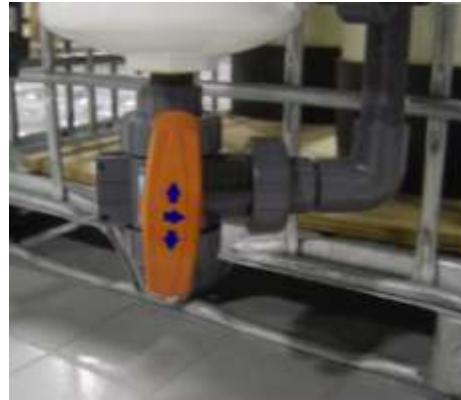
Figure 5: V9 in Position 2
