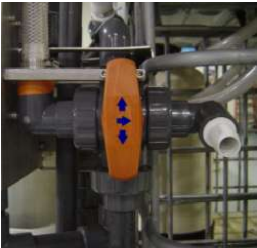
Figure 2: V6 in Position 1
