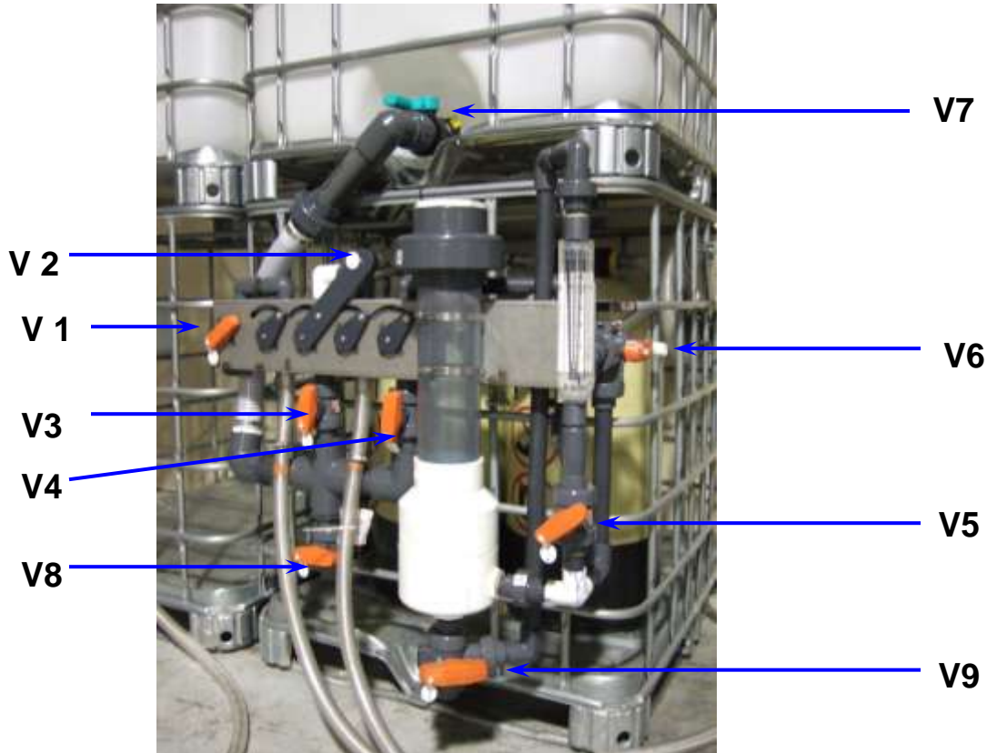
Figure 1: Valve settings at startup
